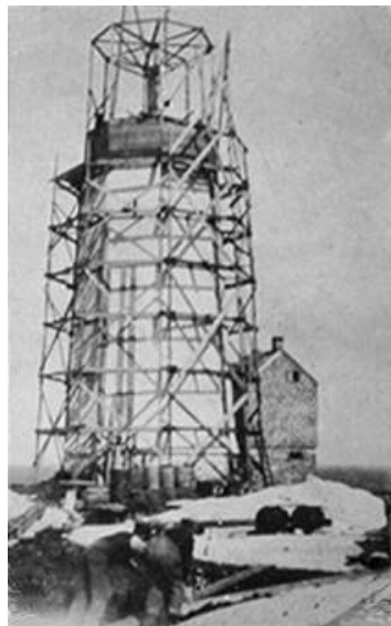
The beginning of the concrete addition of 1906. The vertical arrangement in the center of the concrete may be the shaft for the clockwork weights. Use of salty beach sand to make the concrete caused the gallery to fail 90 years later. Photo courtesy of the NSARM.
